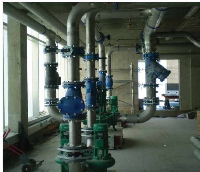
The practised eye will appreciate how the light weight of stainless-steel pipework in this chilled-water rooftop plant room can reduce installation time compared with carbon steel — perhaps making it three times quicker — by virtue of features such as it being much lighter in weight and quicker to weld.
